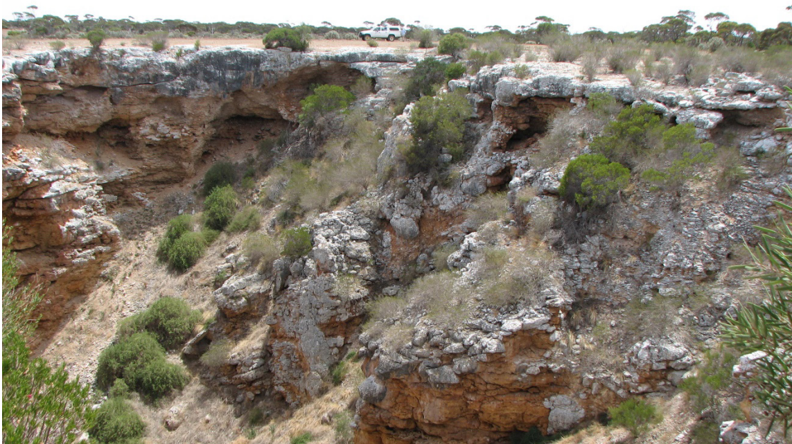
Image: Chowilla Landslip collapse doline, photo K. Dixon
